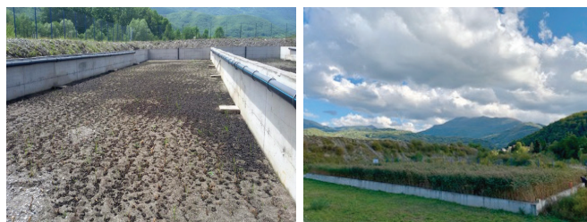
Fig. 2 – Sludge drying reed beds at the finalisation of construction works (left), and after the first year of operation (right) (source: LIMNOS Ltd.)
