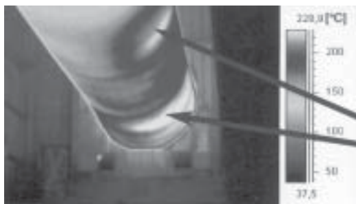
Fig. 4 — Breakdown of refractory on a rotary cement kiln
